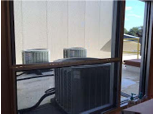
8. Rooftop Mechanical Equipment
